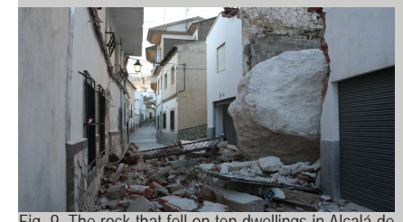
Fig. 9. The rock that fell on ten dwellings in Alcalá del Júcar.
