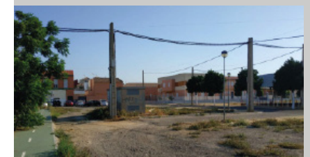
Fig. 9. Existing transformer station (Detailed Study).
